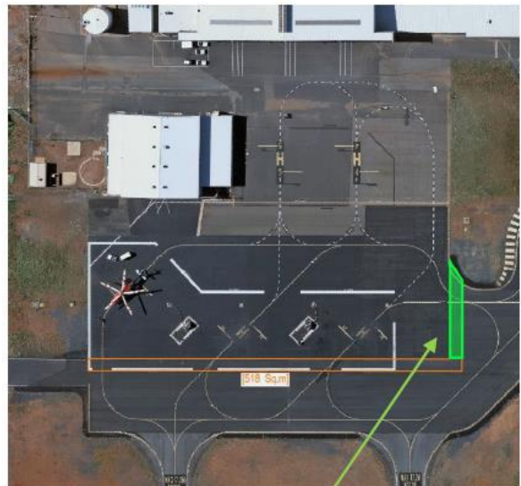
Figure 9. P2 – Taxiway Asphalt Joint (Section 3). *To complete after Viva Fuel Line Scope
